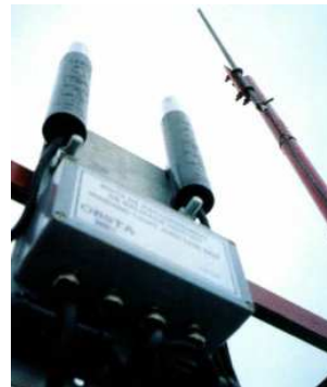
Obsta Solar Power Supply
